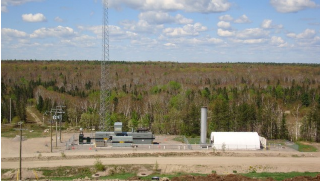
Figure 4: Landfill Gas Utilization to Electricity Facility and Landfill Gas Flaring Station located at the City's Merrick Landfill Site
