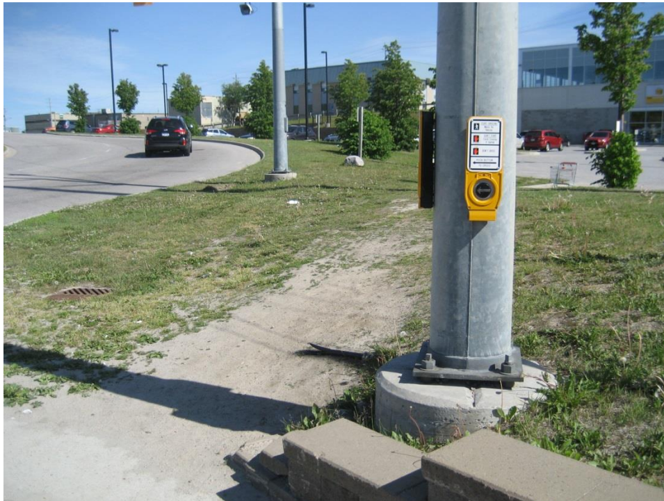
Sidewalk not provided to a pedestrian destination, Josephine Street & McKeown Avenue
