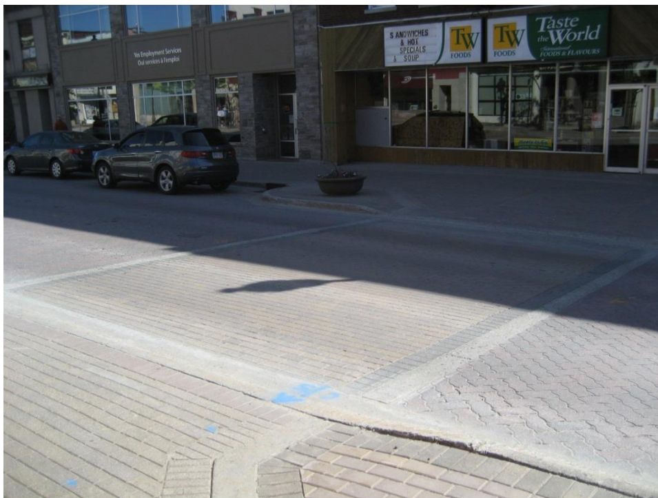
Pedestrian crosswalk not marked with eye-level signage, Main Street
